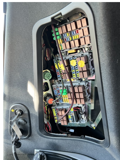
Figure 2.25. CANBUS Cable termination.
